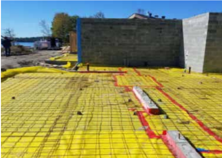
View from end of Unit No.5 towards Unit No.4 Stego Wrap Vapour Barrier with 152x 152 6/6 Wire Mesh
